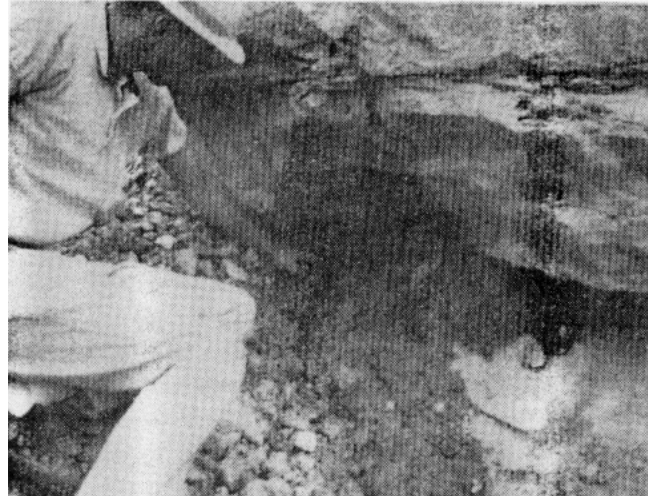
Figure 3-10. Seepage from spring in abutment at Green River Dam, Kentucky
