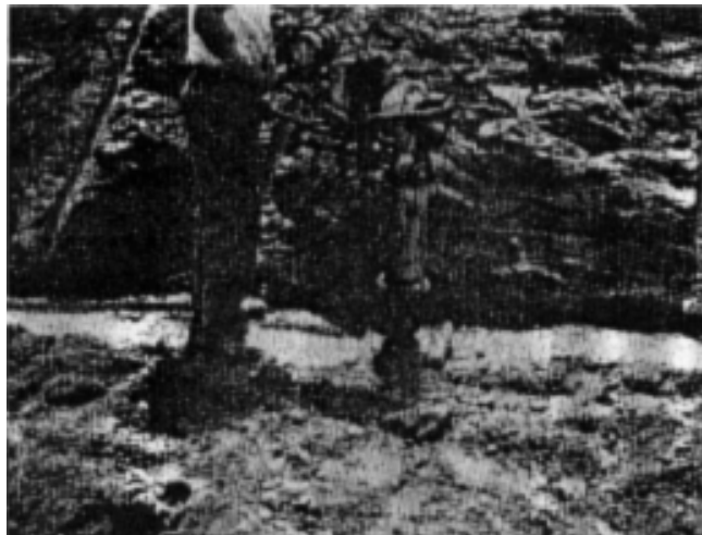
Figure 5-12. Compacting against rock abutment with a hand-operated power tamper, Green River Dam, Kentucky
