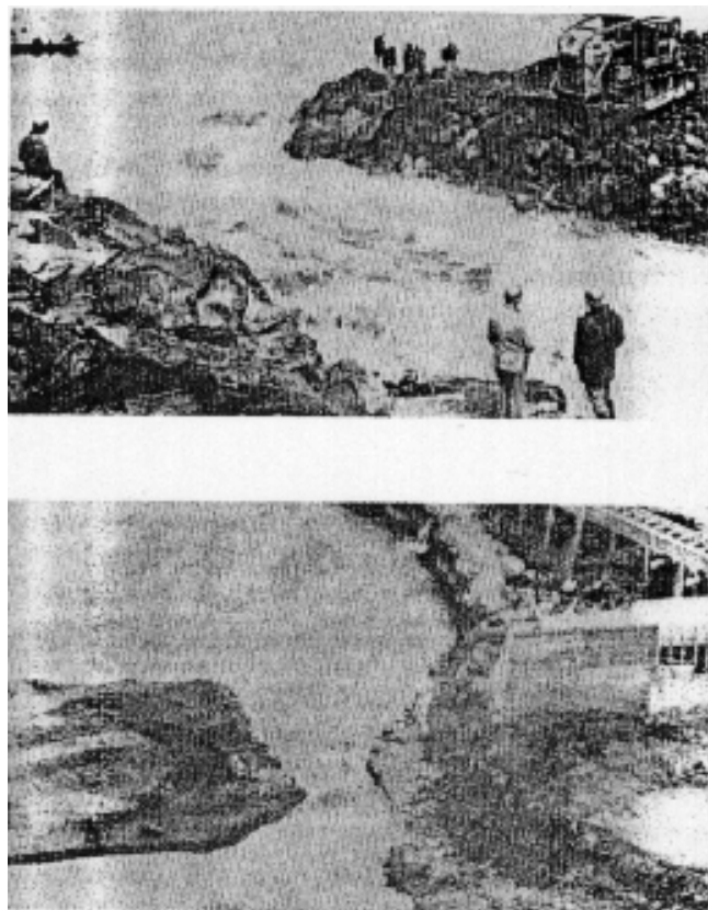
Figure 6-1. Examples of end fill closure method. (a) River closure, cofferdam, Mica Dam, British Columbia; (b) two days before final closure, Dalles Closure Dam, Columbia River
