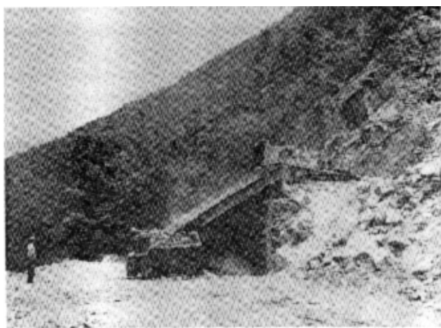
Figure 4-6. Rock separation by means of a sloping bar (grizzly) arrangement at Gathright Dam, Virginia
