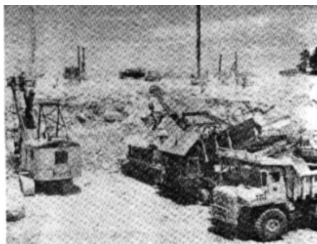
Figure 4-7. Grizzly wobbler discharging +2-in. rock into end-dump truck and -2-in. material into bottom-dump truck (spillway-powerhouse excavation at Stockton Lake Dam, Missouri)
