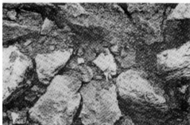
Figure 5-5. Test trench through portion of rock test fill at New Melones Dam, California. General view of trench (top); closeup view of trench wall (bottom)
